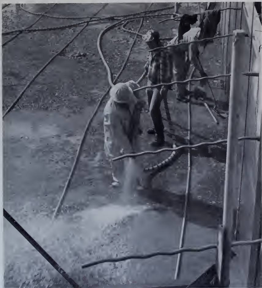
Figure 122.—Final washing with water jets just prior to placing next lift of concrete. P1222-142-11967.
